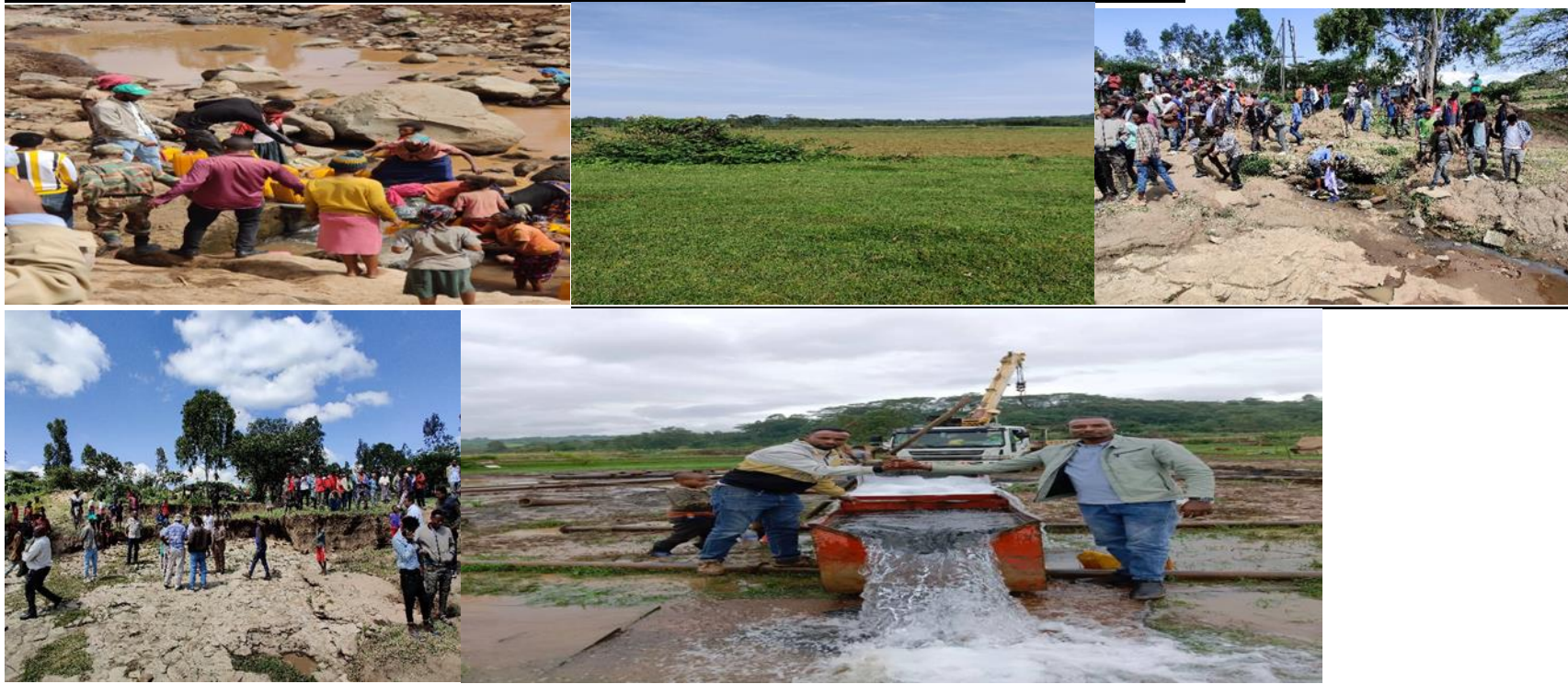
Pictures of the selected sites for rehabilitation of water systems infrastructure and drilling of boreholes in Bashasha and Adilo
