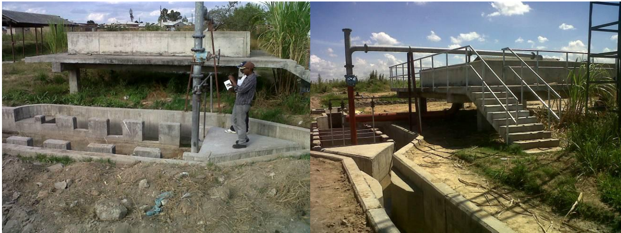
Pump Station 3 Vertical Flow Grit Chamber & Decanting Chambers before and after rehabilitation (photos 24 & 25)
