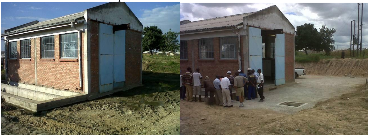
Pump Station 3 drainage and offloading bay pavement and drainage before and after (photos 22 & 23)
