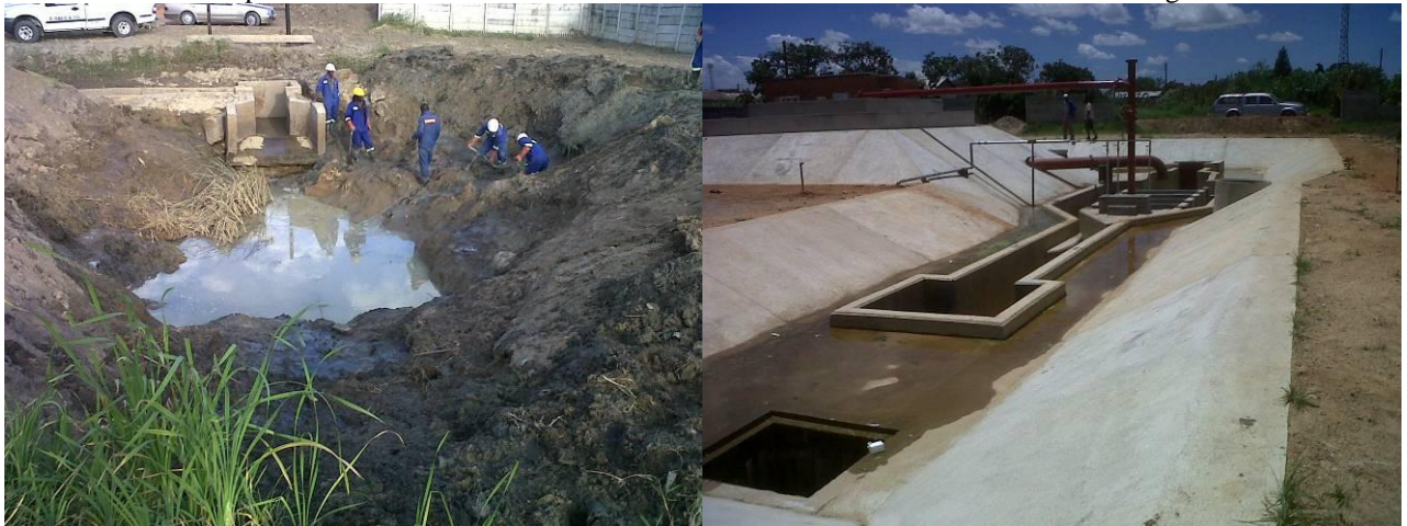
The Vertical Flow Grit Chamber used to trap sand before (photo 5) and after completion (photo 6)
