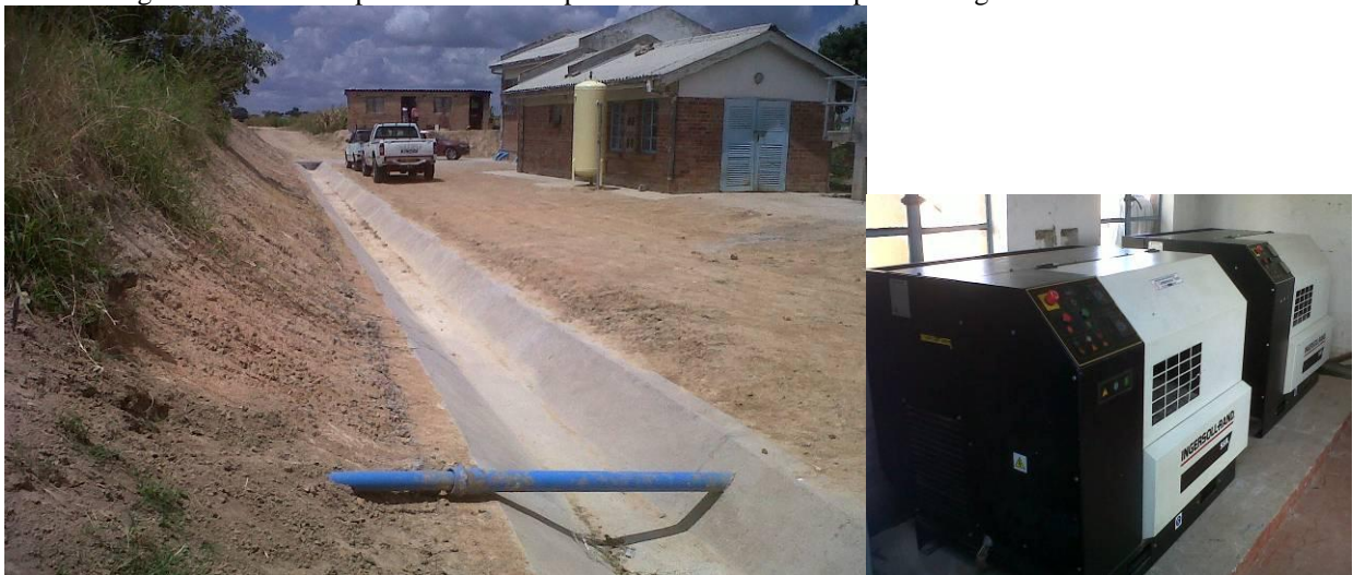
Pump Station 3 refurbished building and pressure vessel with new surface and subsurface drainage facilities (photo 20) Photo 21 shows the rehabilitated compressors
