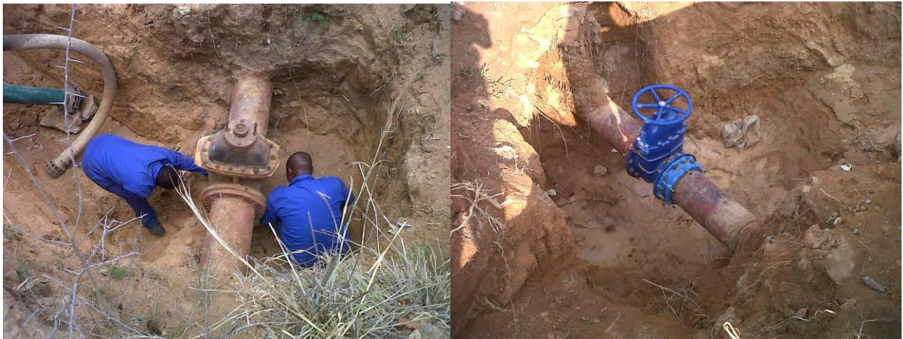
Photo 4 & 5 show replacement of old non functional control valves needed for water demand management
