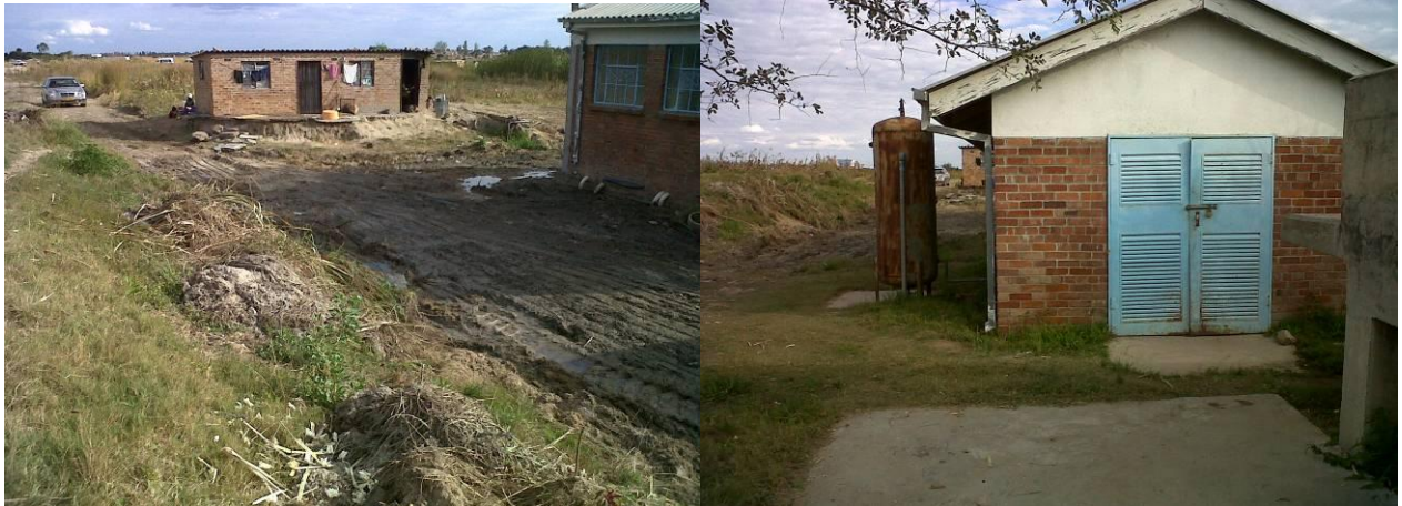
Existing Pump Station 3 building and attendant's house showing waterlogged ground condition (left photo 18). Photo 19 on the right shows the compressor room and pressure vessel used to operate the grit removal mechanism.
