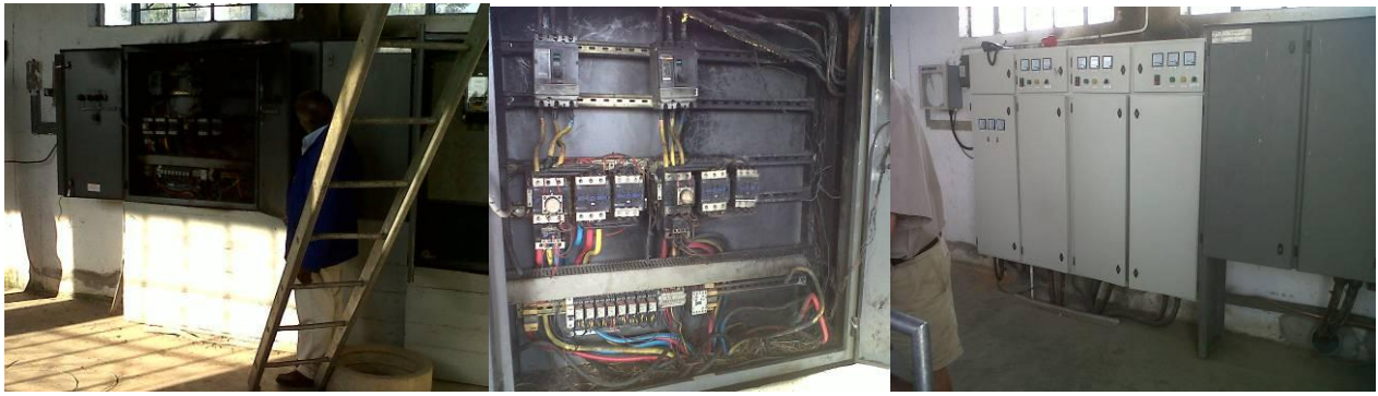
Existing burnt out pump control gear – left (photo 15 & 16) and the new replacement control gear (photo 17)
